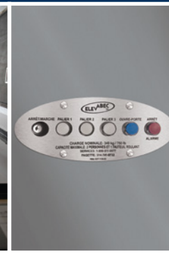
Remote control in the cabin
